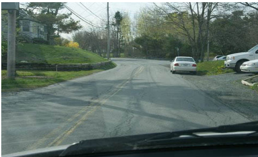
Figure 2. Cobequid Road narrow shoulder sections inhibits complete off-road parking and requires pedestrians to walk around parked vehicles by stepping out onto the paved road. The lack of safe walking areas along this part of the Road has required that school children be bused to the Waverley Memorial Elementary School.
